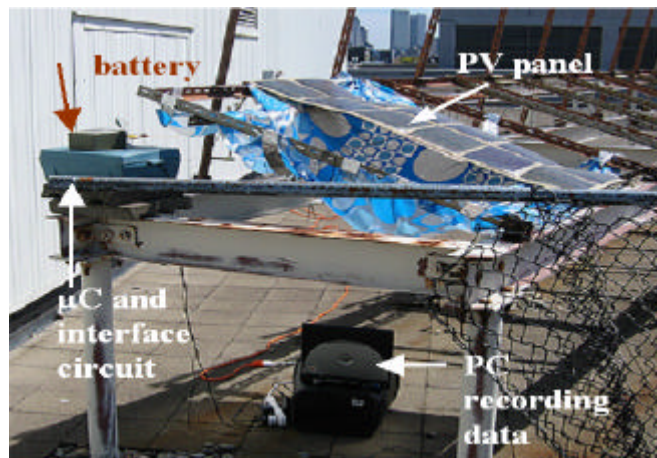
Figure 3: Experimental set-up on rooftop. The 12 V NiMH battery is charged by a solar array and is connected to a prototype battery charger with microcontroller (The size of the box is not at all related to the size of the circuit).
